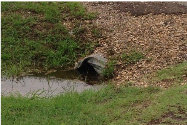
Figure 6D: Damaged Culvert Example
